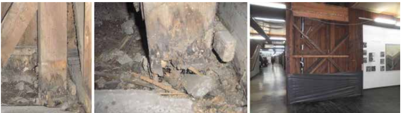
Figure 9. Severe damage to central frame columns
