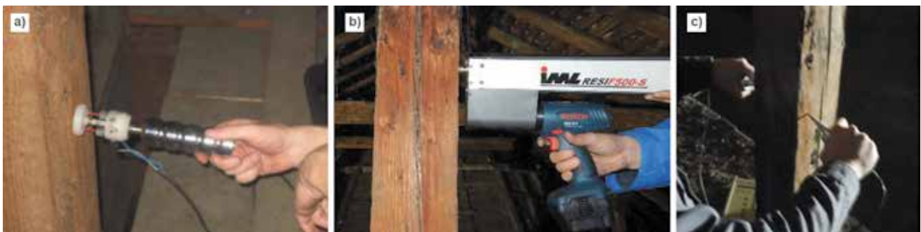
Figure 10. a) Measurement of moisture content, b) drilling with the resistograph device, c) ultrasound measurements
