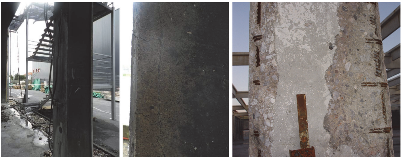
Figure 5. Column damage by fire: a) column blackening; b) cracking; c) exposed reinforcement
