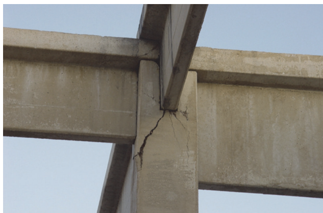
Figure 7 Damaged details at the beam – column connection
