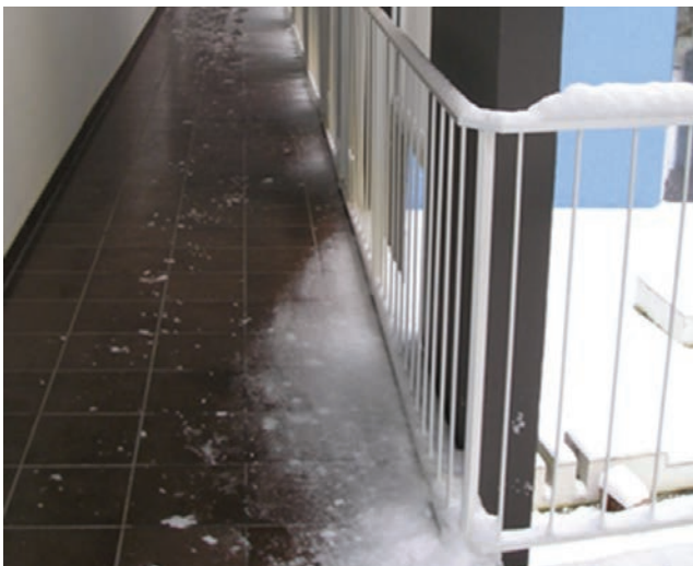
Figure 14. Faulty gallery design, Source: MCPP, [5]
