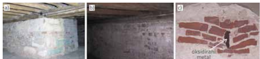
Figure 3. Masonry details from the palace: a) basement; b) second floor; c) damage due to oxidation of a metal clamp inside the wall
